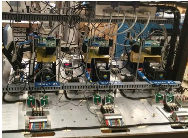
Figure 10: Low Power Test Bed Power Hardware
