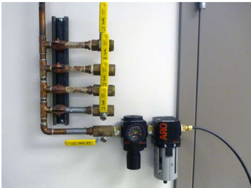
Figure 5: Compressed air turned on (bottom valve).
