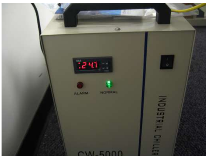
Figure 3: Water chiller up and running at 24.7 degrees C.
